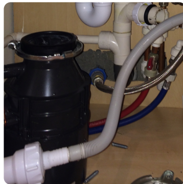
Caption Insinkerator to be removed
